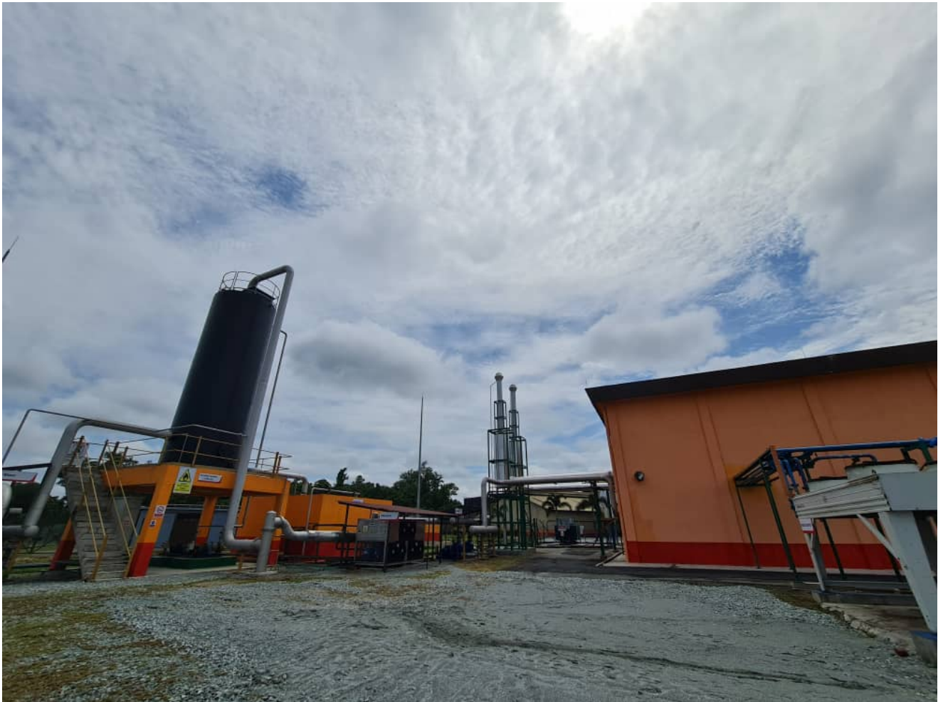
FGV's Triang biogas power plant building
